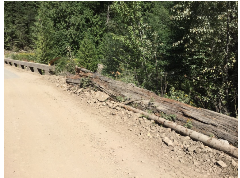
Fender at upstream left bank
